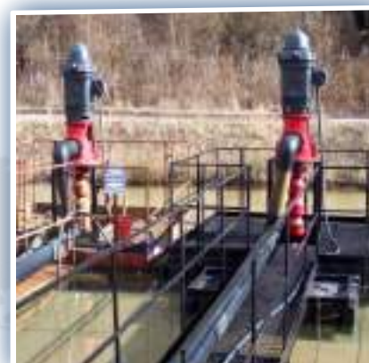
Mine Dewatering Pump
