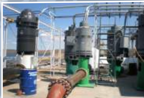
Pump Used for Portable Irrigation
