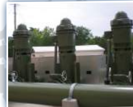
Deep Well VTP Pump
