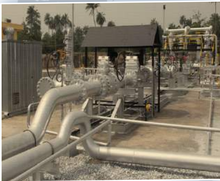
Gas Metering System
